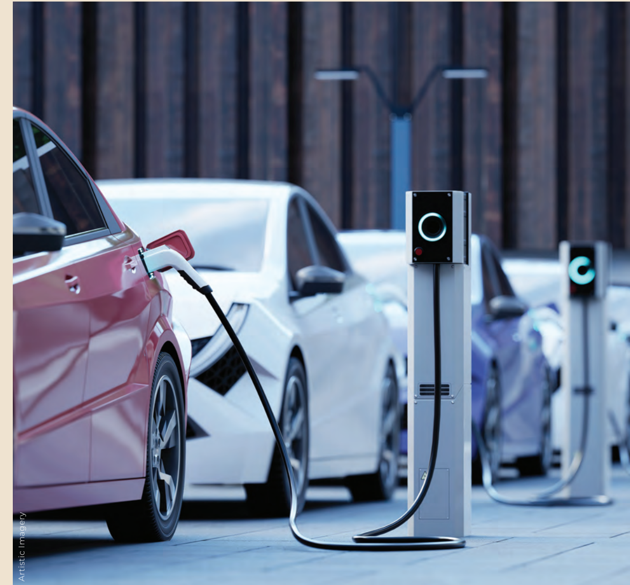
EV Charging Stations
